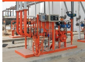
19 BLENDING, METERING AND LOADING SKID
