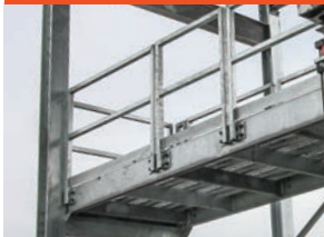
12 METAL HANDRAILS AND CUSTOM PLATFORM
